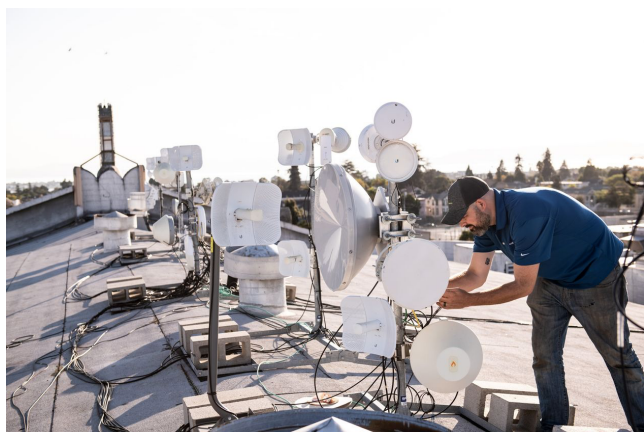
Jonathan Weinberg of Common Networks inspects an antenna installed on the roof of the Alameda Theatre and Cineplex, the tallest building in Alameda, Calif. PHOTO: WINNI WINTERMEYER FOR THE WALL STREET JOURNAL
